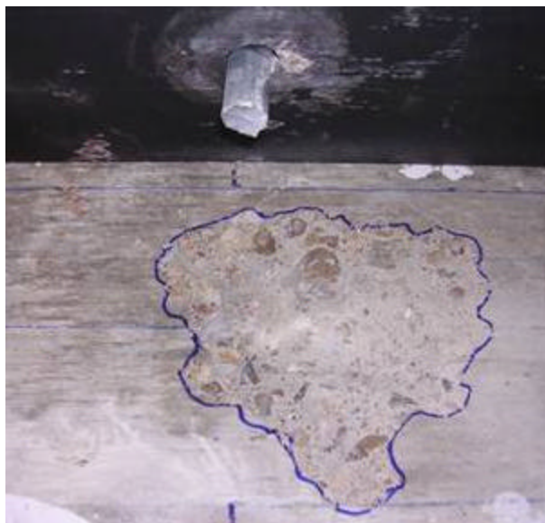
Figure 5.46: Failed Specimen WEDGB25
