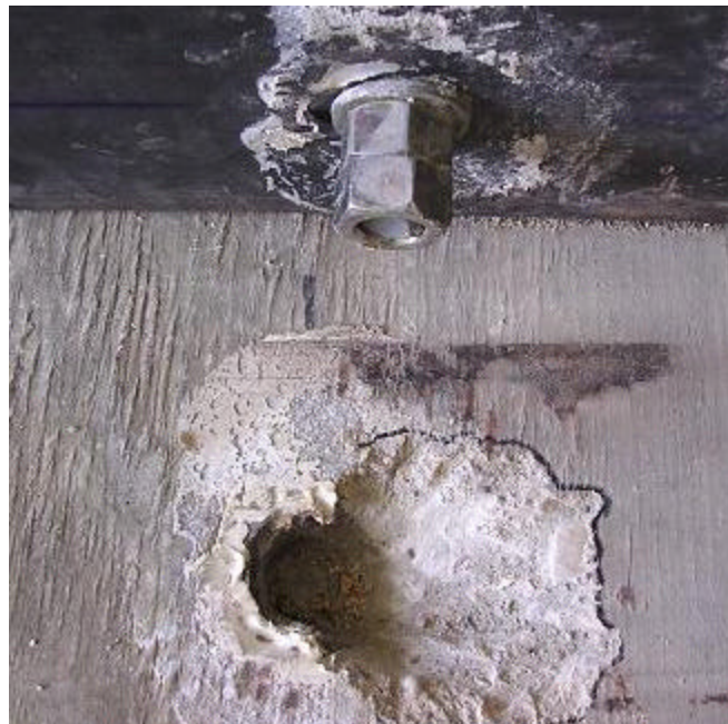
Figure 5.37: Failed Specimen DBLNB60
