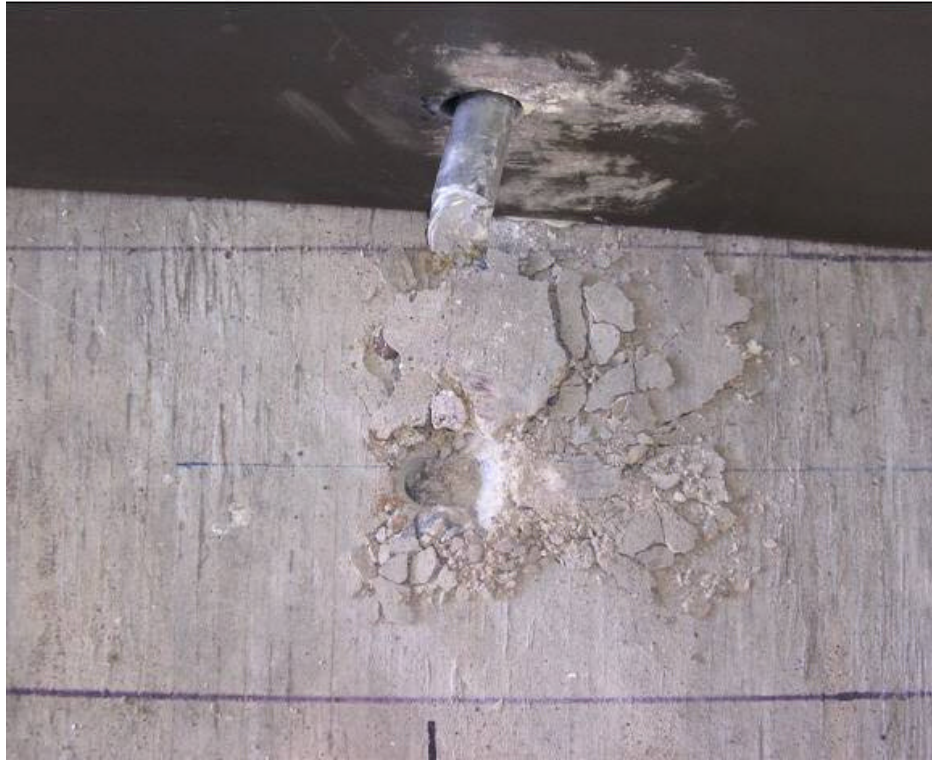
Figure 5.23 Failed Specimen WEDGB-ST
