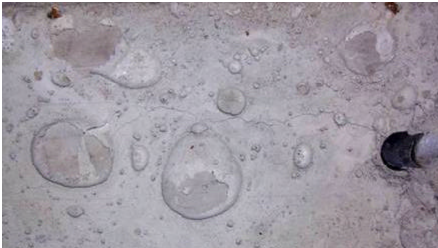
Figure 5.3: Voids and longitudinal crack behind stud (Specimen CIPST-ST)
