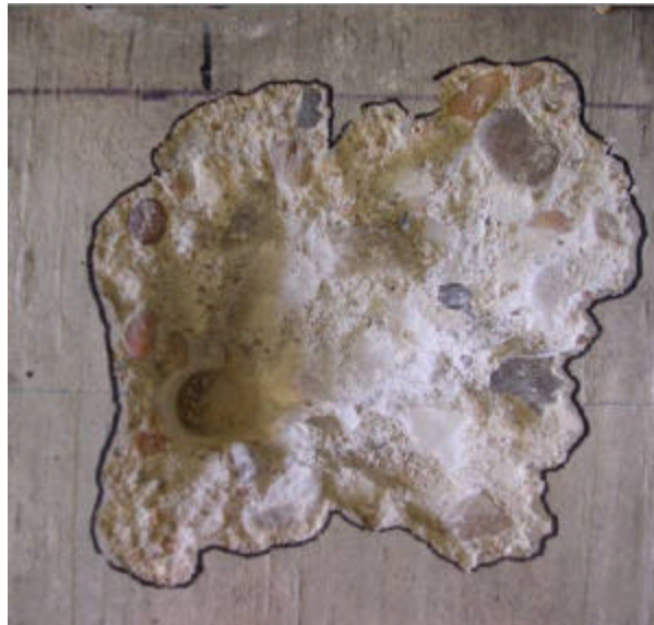
Figure 5.24 Local crushing of concrete (Specimen WEDGB-ST)
