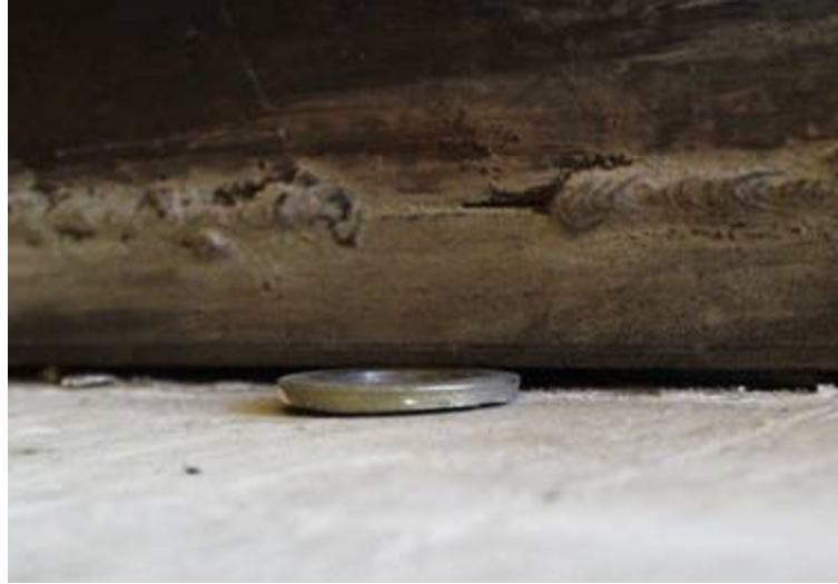
Figure 5.5: Gap between steel plate and concrete block (Specimen POSST-ST)
